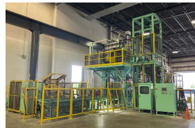
Container Exchanger and Course Grinder
